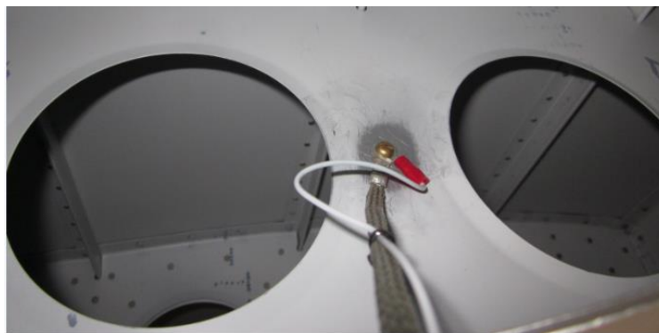
Figure 10: Bonding strap and earth lead of connector attached to Rib no. 16.
